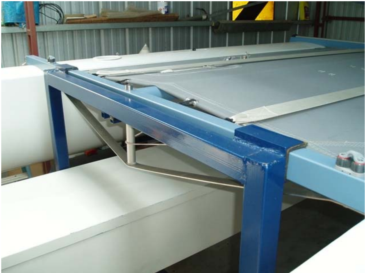
Main beam support
